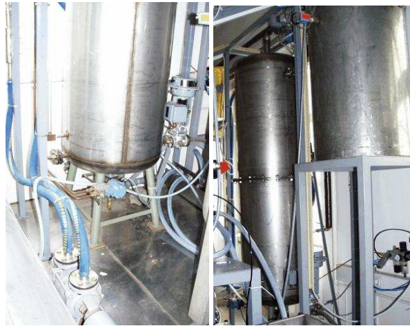
Figure 5.1: The gas-liquid separator part of the process plant at the Jozef Stefan Institute (Slovenia). A pump feeds the gas-water mixture into a reservoir where the gas is separated from the water.
